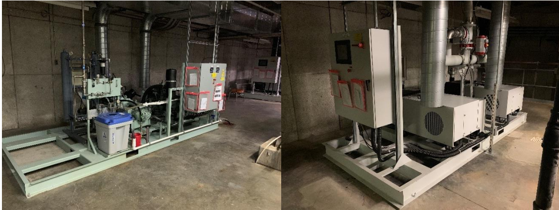
Figure 6. Compressors (left) and Vacuum Pumps (right)
